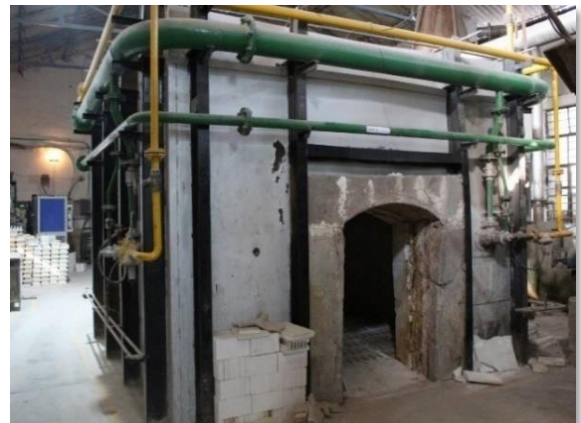
Kiln -D (7 ton)- natural gas fired downdraft firing the material
