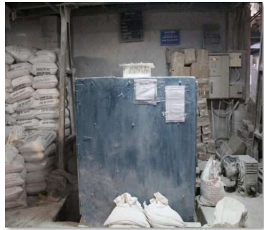
Ball mill-2 – for crushing raw material into powder
